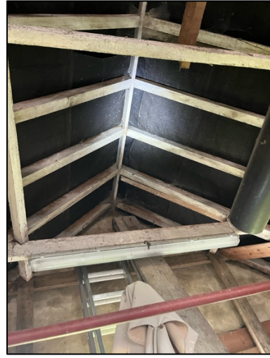
Photograph 25. The bitumen lining with rips and tears throughout, providing access to the roof tiles.
