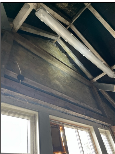
Photograph 22. The southern side of the roof from the inside of the shed, showing access points at the roof apex.
