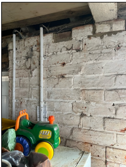
Photograph 16. The main brick walls inside the property. Missing bricks at the top, allowing access to the eaves.
