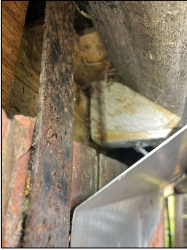
Photograph 18. Further photograph of the metal plating over the eaves, gaps on the sides allowing for easy access.
