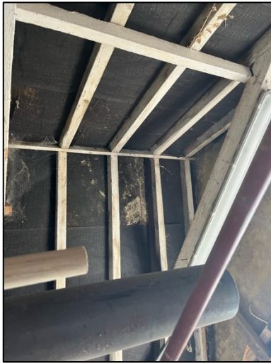
Photograph 24. The bitumen lining with rips and tears throughout, providing access to the roof tiles.
