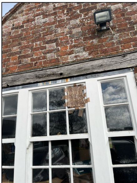
Photograph 5. The window on the southern side of the property, a closer view of the wooden board surrounding the top of the window, with a large gap
