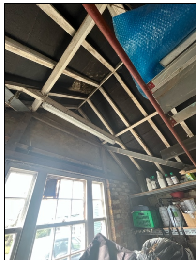
Photograph 23. The southern side of the roof from the inside of the shed, showing the window providing natural lighting.
