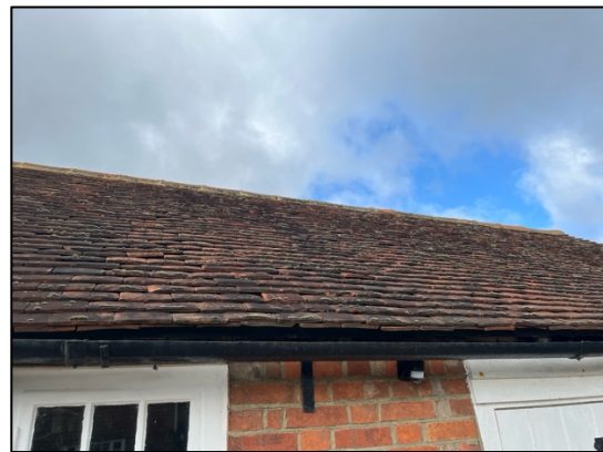
Photograph 9. The roof of the building from the east side; showing the gaps between the roof tiles.
