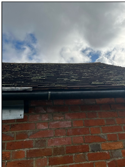
Photograph 10. The roof on the west side of the building, showing gaps between the roof tiles.
