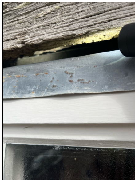
Photograph 6. The same gap between the window frame and the wooden board, torchlight to show the depth of the crevice.
