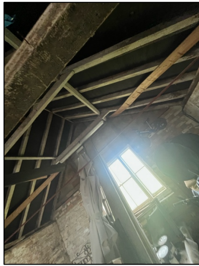
Photograph 21. The northern side of the roof from the inside of the shed, with a window providing natural light.
