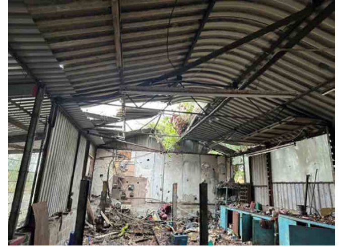
9. Photo taken within the steel frame barn to be removed from site.
