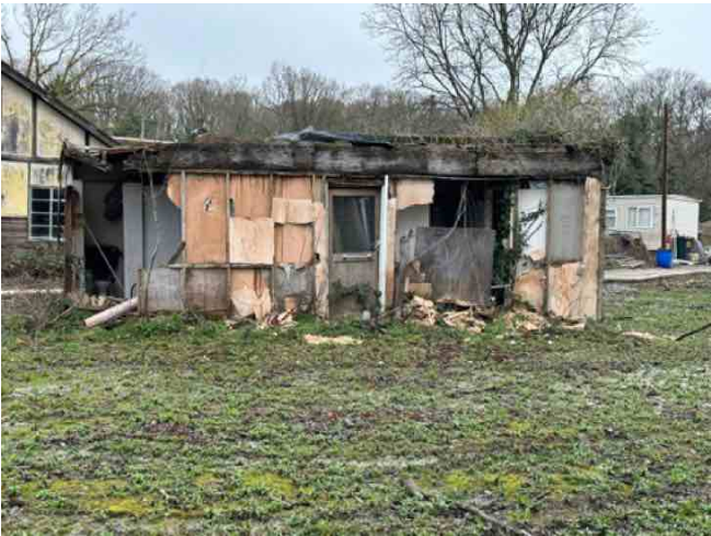
10. Existing outbuildings in disrepair.
