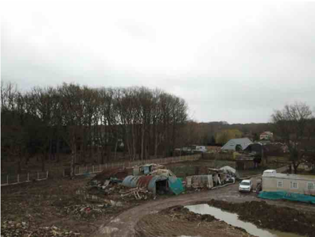
16. View taken from the centre of the site looking towards Cherrytree Paddock and boundary
