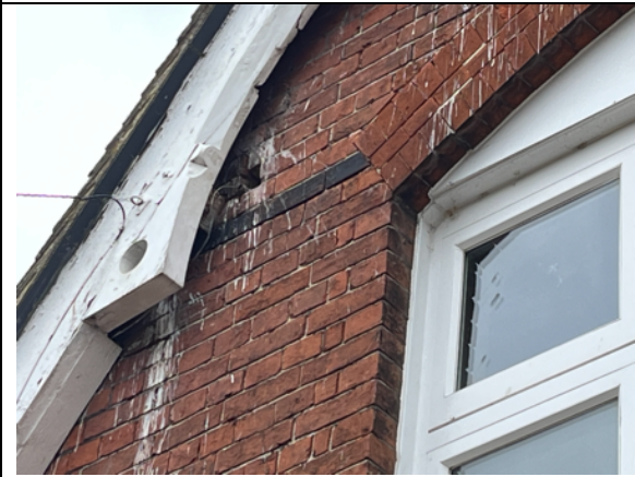
Photo 5. Hole in brickwork to east elevation of northern section of building, where starling was nesting – note abundant bird dropping evidence, indicating frequent and intense use by nesting birds
