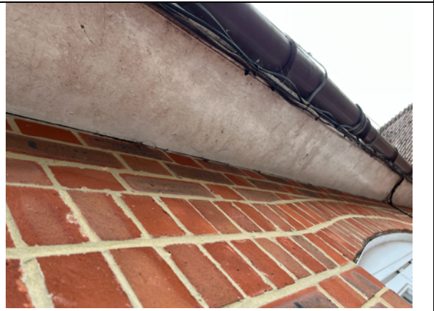
Photo 6. Tight-fitting soffits to western aspect of main building, with cobwebs evident in few very narrow gaps
