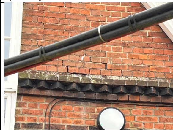
Photo 7. Brickwork cracks on north-east elevation of main building, found on close-inspection to be too shallow (<3cm) to support roosting bats
